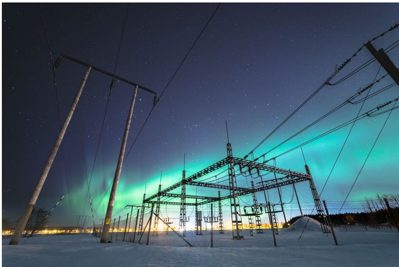
Northern Lights (Aurora borealis) and outdoor electrical switchgear at winter night, snow field. By Alexandr Patshin, Shutterstock: https://www.shutterstock.com/image-photo/northern-lights-aurora-borealis-outdoor-electrical-1081616435
