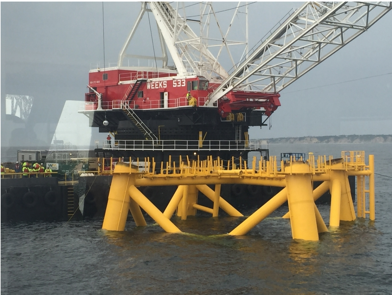
The foundation of one of the five wind turbines being built three miles off the southwest shore of Block Island is under construction on July 27, 2015, the day town, state and company officials visited the site by boat for a ribbon-cutting ceremony. (Ken Lacoste/Special to The Day)
