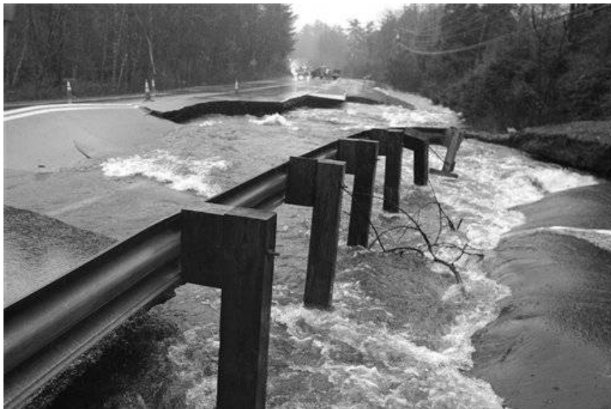
Photo – msnbc.com April 16, 2007 – Heavy rains wash away a section of Route 4 in Nottingham, NH
