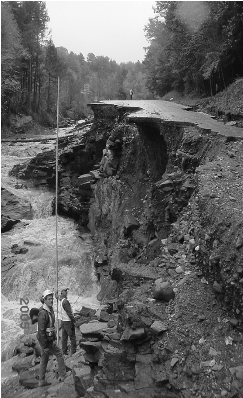
Photo #5. Route 123 washed out – roadway embankment fill, underlying soil and fractured rock stripped to bedrock at location west of Route 12-A intersection. (Photo by Dick Lane – NHDOT.)
