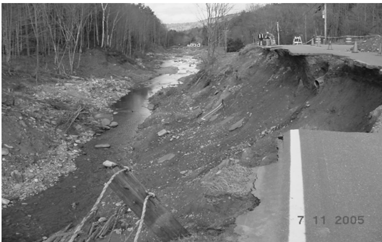
Photo #1. Route 123 washed out by floodwater at the intersection of Cooper Hill Road. (Photo by Dick Lane – NHDOT.)
