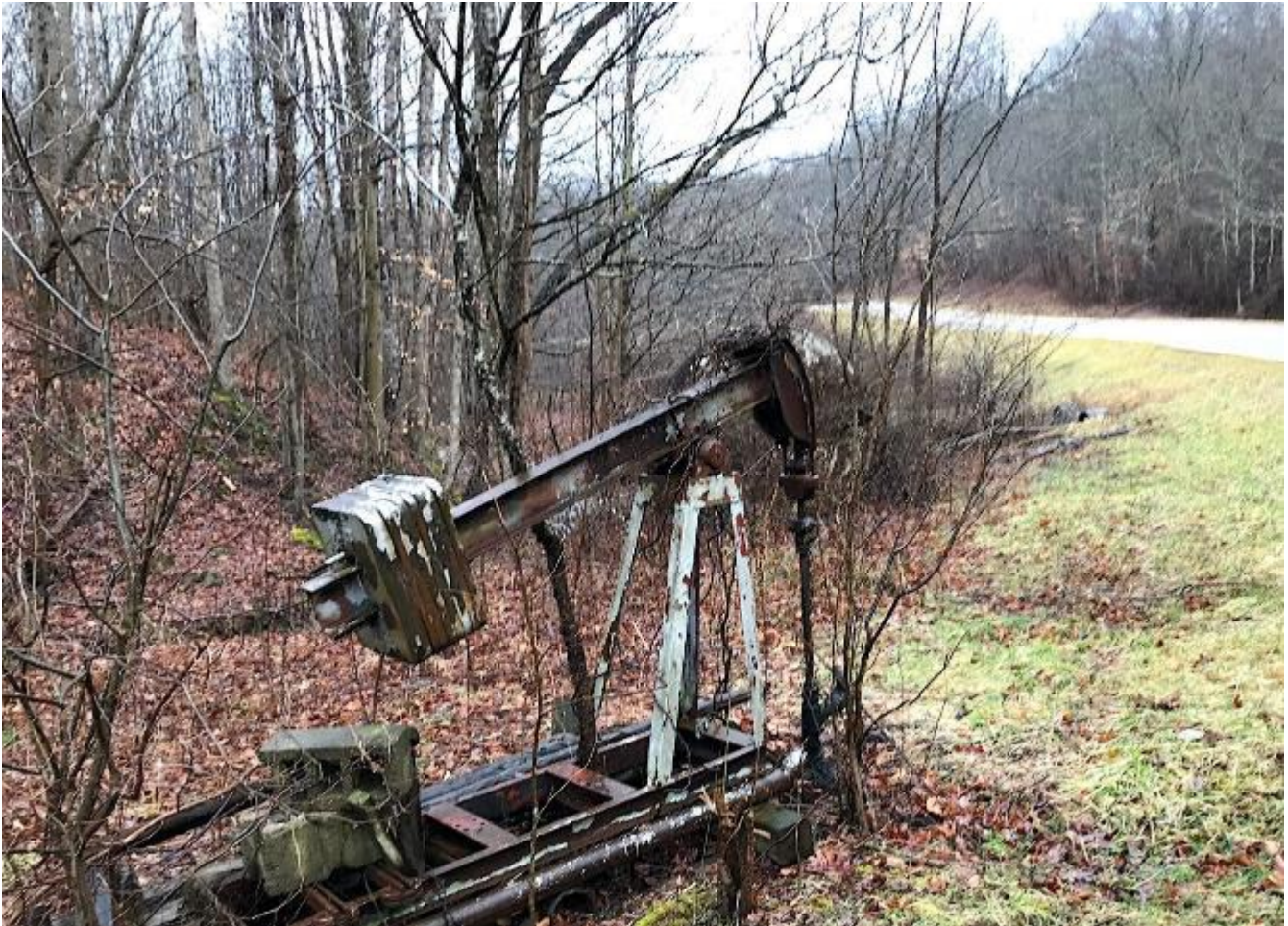
This abandoned oil well, dating back to the early 1900s, was finally plugged in September 2020. Credit: Ohio Department of Natural Resources
